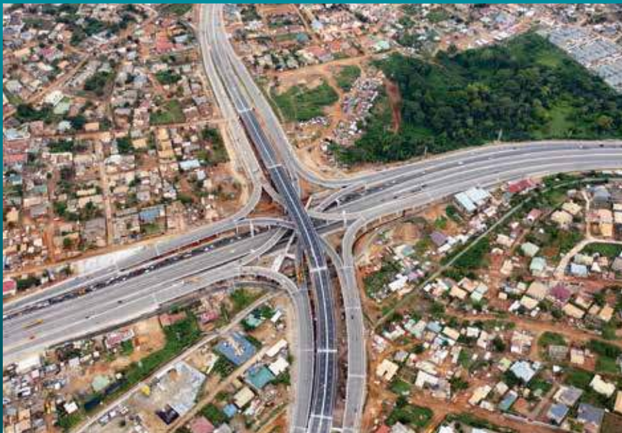
Construction of road in Ghana, part of the Ghana-Burkina Faso Road Corridor
